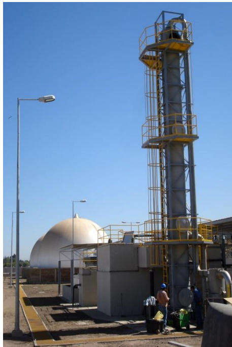
Biogas washer system
