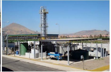
Biogas washer system
