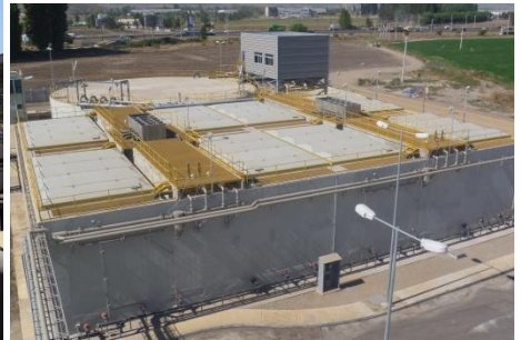
UASB anaerobic reactors
